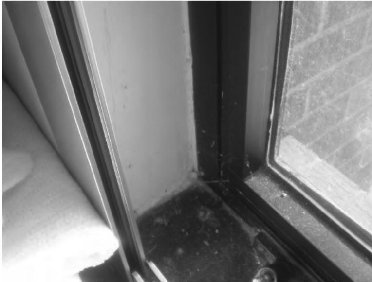
Window Caulk Sample G - 19A
