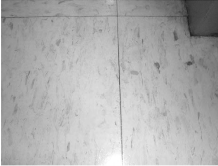
9"x9" Red Vinyl Floor Tile (under exposed white vinyl floor tile) Sample 4 - 17A
