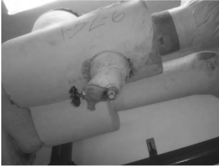
Pipe Elbow Insulation Sample 3 - 22A
